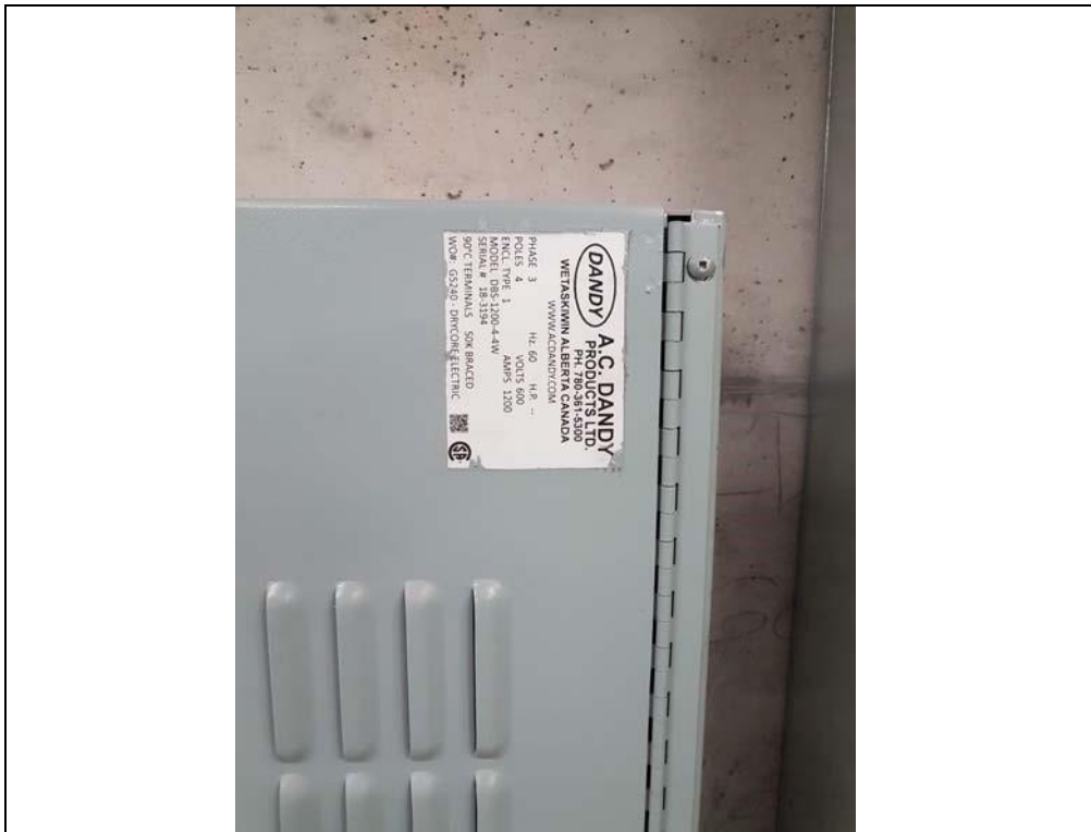
BUS BAR SPLITTER TROUGH A.C. Dandy, DBS-1200-4w.
